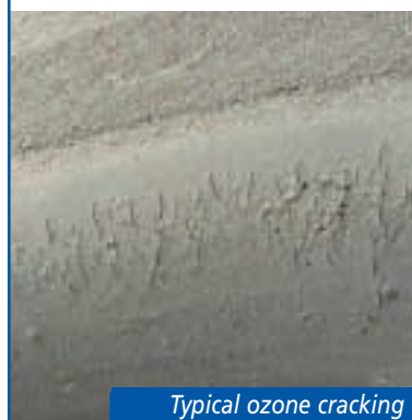
Ozone cracking in groove
